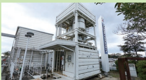
Waste water regenerating system
